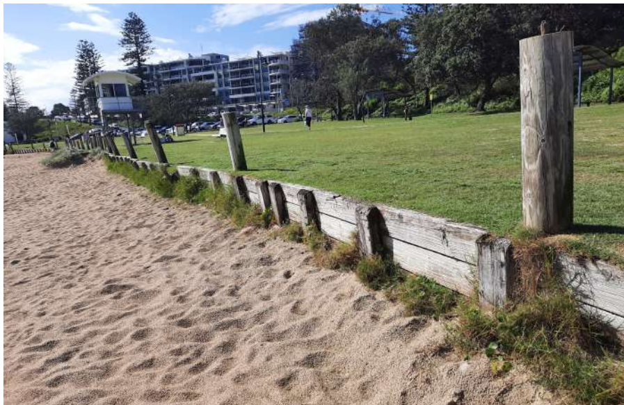
Seawall - nearing end of life replacement
