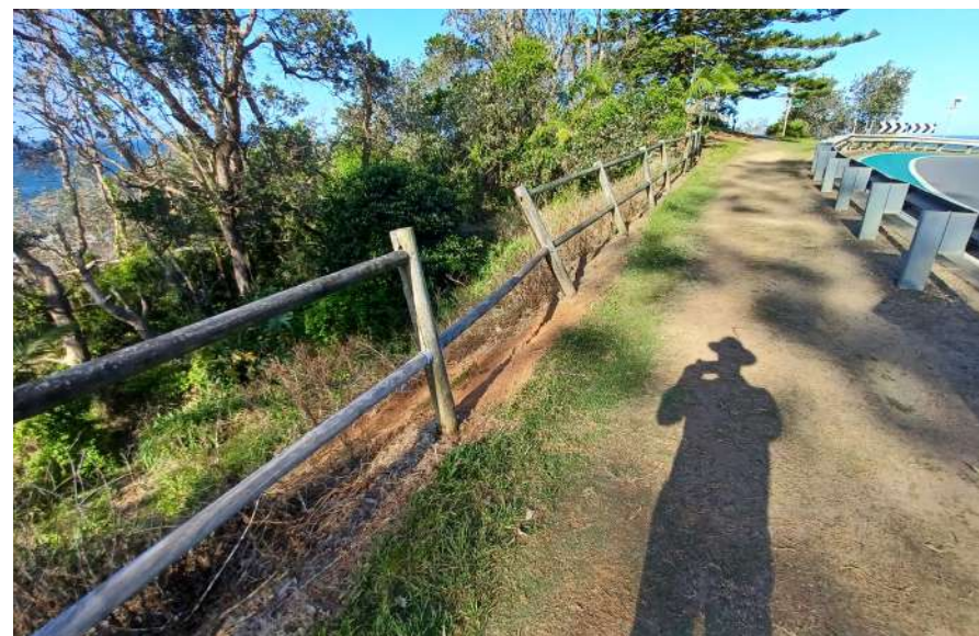
fence in disrepair along William Street
