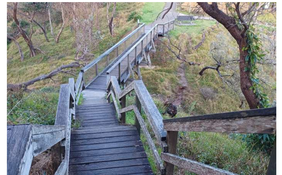
Bridge/boardwalk near end of life replacement
