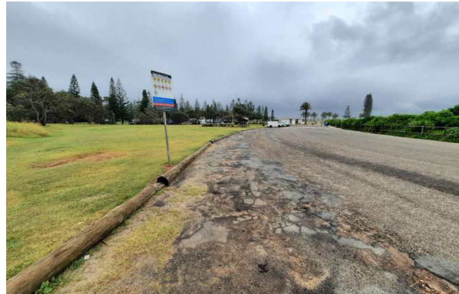
Northern carpark in poor condition
