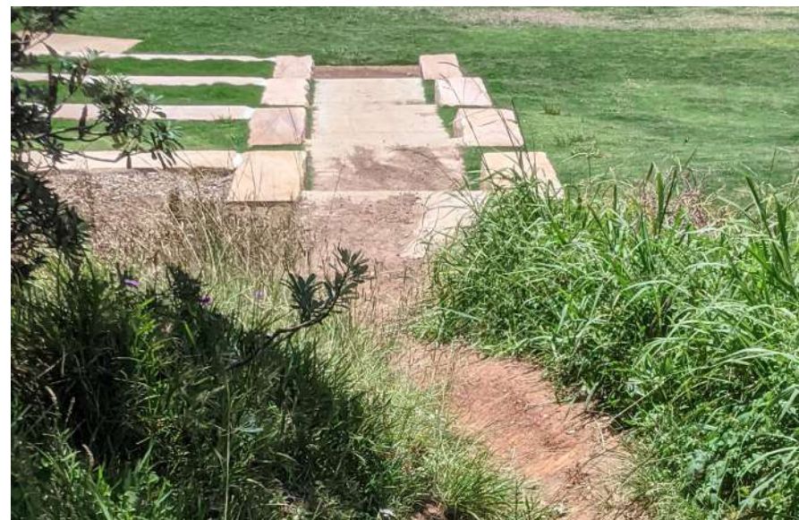
Eroded track to amphitheatre from lookout
