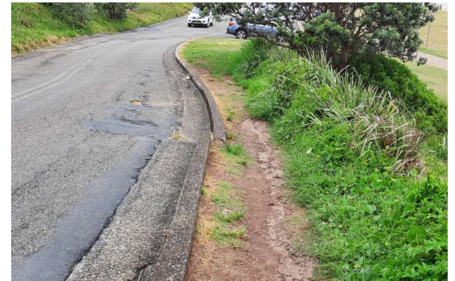
Eroded track along Alban Place
