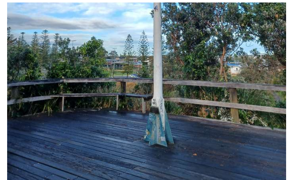
Lookout - nearing end of life replacement
