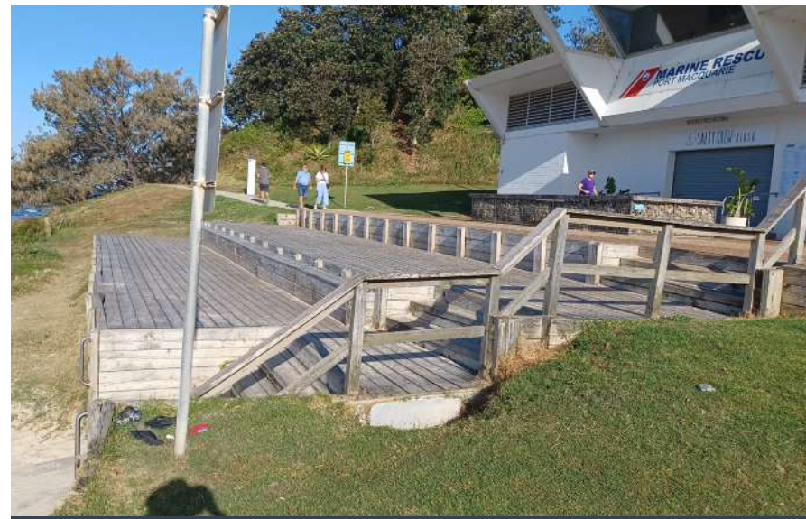
Deck - nearing end of life replacement
