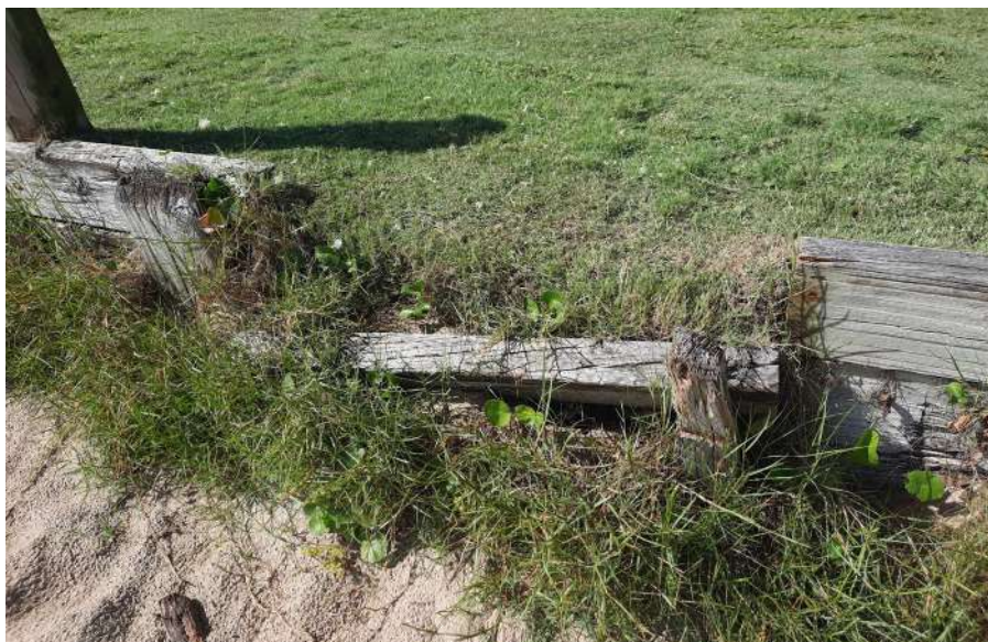
Seawall - partial collapse
