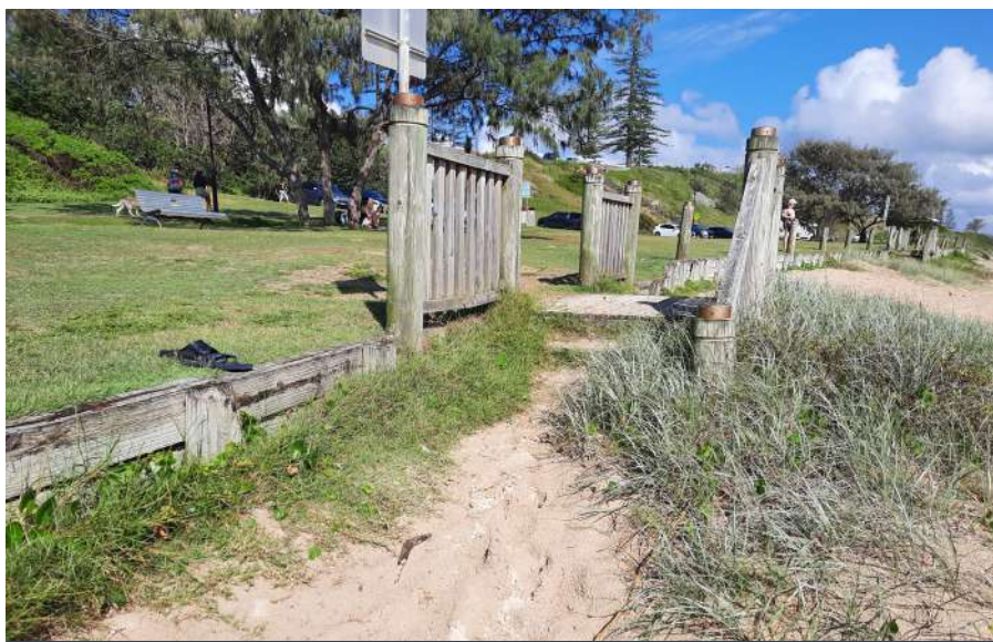
Seawall stairs in poor condition
